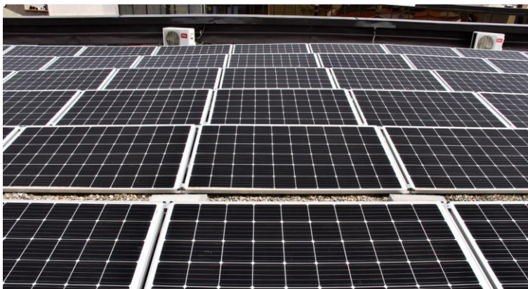
Solar Panels at Municipal Administrative Building in Prizren ©UNDP, 2021, T. Talosh
