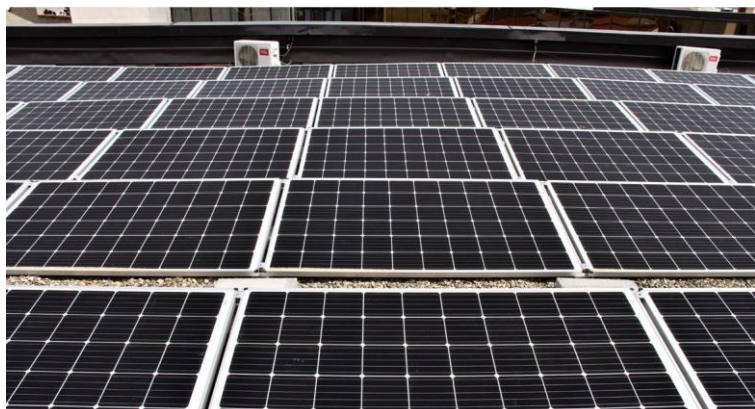
Solar Panels at Municipal Administrative Building in Prizren ©UNDP 2021, T. Lalosh
